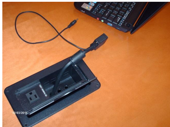
Closeup of VGA and Audio Cable
